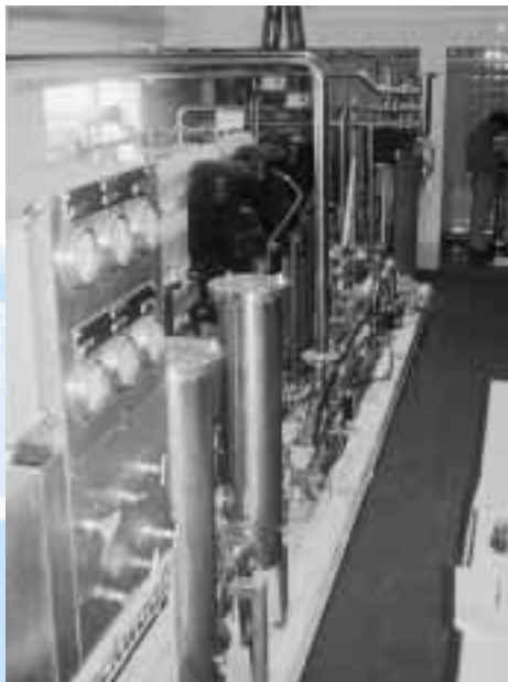
Various SIGNET measurement systems are used in the new reverse osmosis units.
